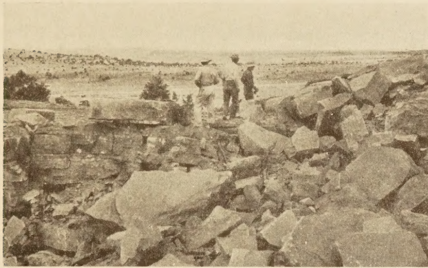
FIGURE 3.—UNDER AVERAGE HIGHWAY CONDITIONS POOR BLASTING SUCH AS THIS IS LIKELY TO INCREASE THE COST OF HANDLING MATERIAL AS MUCH AS 25 CENTS PER CUBIC YARD
